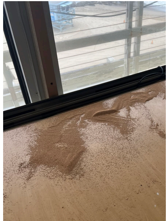
Image 7- Observed Termite droppings
