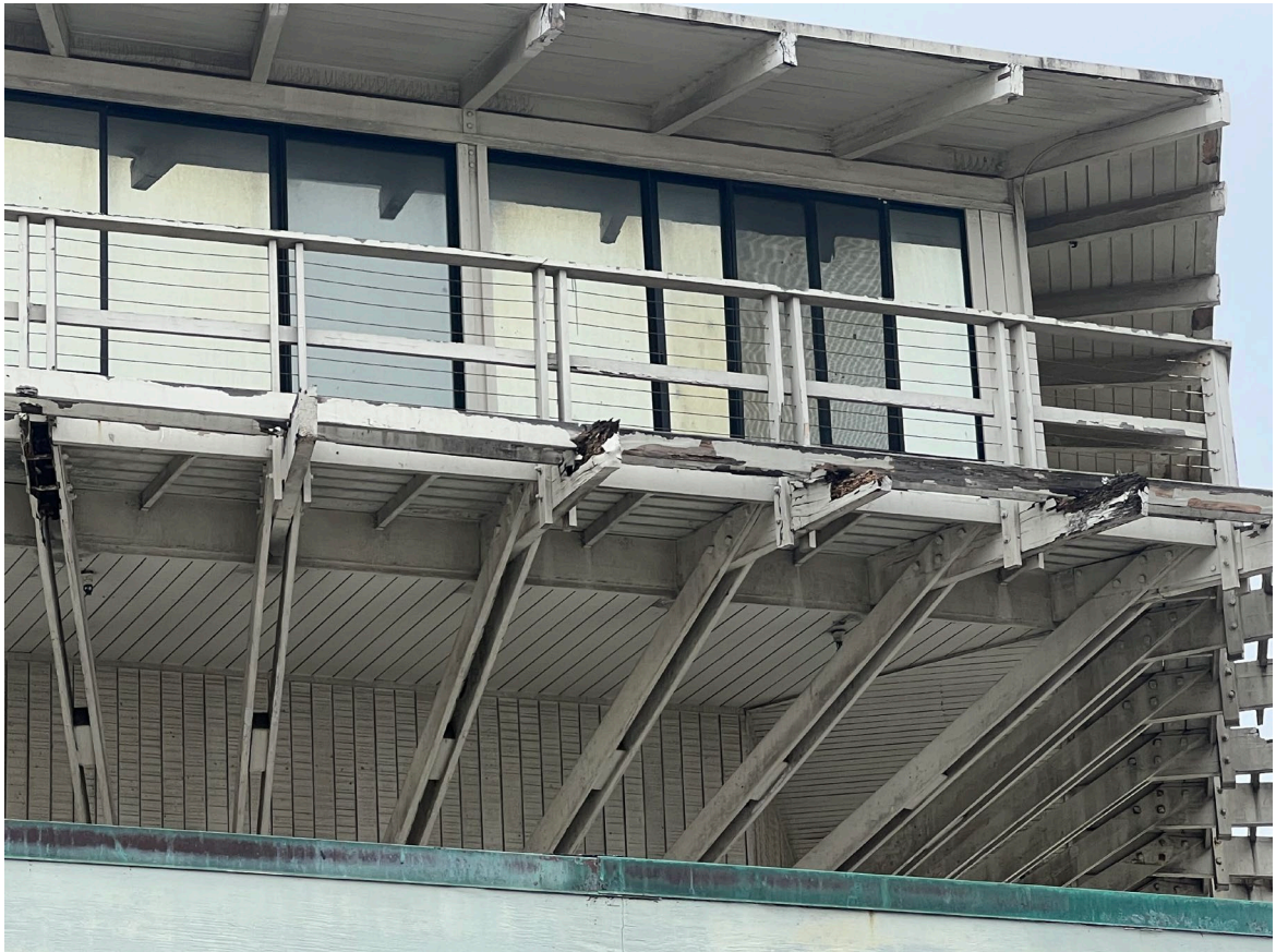
Image 3- Beam damage at 3 rd level balcony
