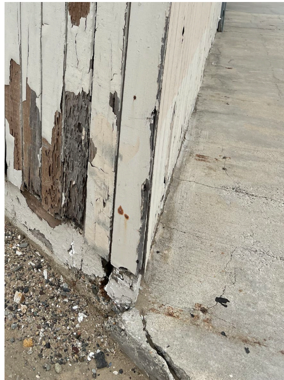
Image 5- Typical Curb and Siding damage
