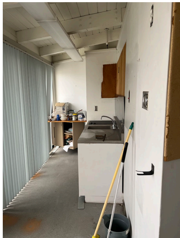
Image 9- Condition at 3 rd level breakroom
