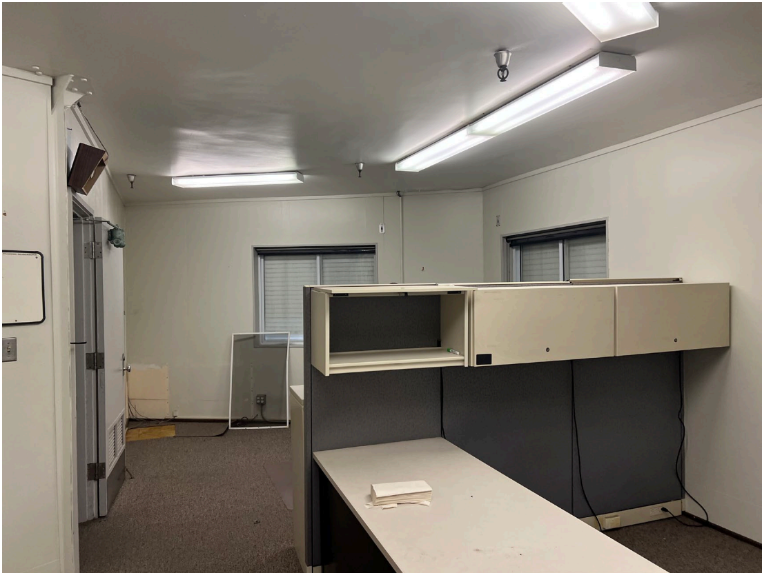
Image 10- Condition at 2nd level office
