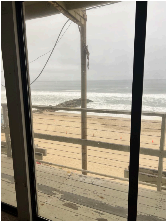
Image 6- Typical Railing/Deck and Beam damage
