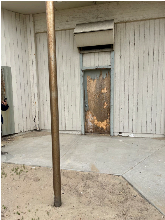
Image 4- Door damage at West elevation
