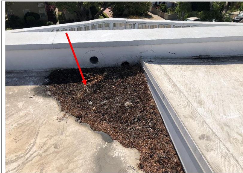
Photo 63: Debris obstructing a drain on the upper roof.
