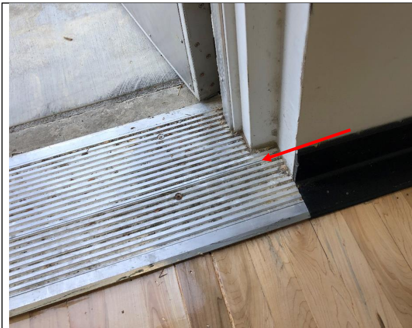
Photo 43: Approved drawings call for a sill pan to be installed under all door thresholds. The sill pan is not visible from the interior.
