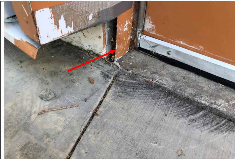
Photo 46: An opening in the sheet metal adjacent to one of the doors.
