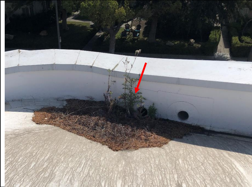
Photo 99: Tree debris built up at scupper drains and along the low parapet. Plants were observed growing in debris on the roof.
