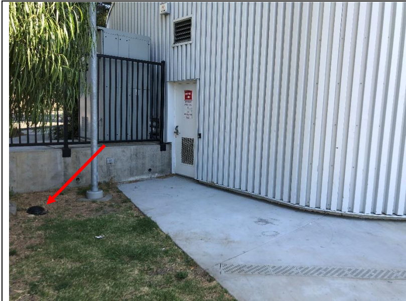
Photo 10: Additional drains had been added in front of entrances.
