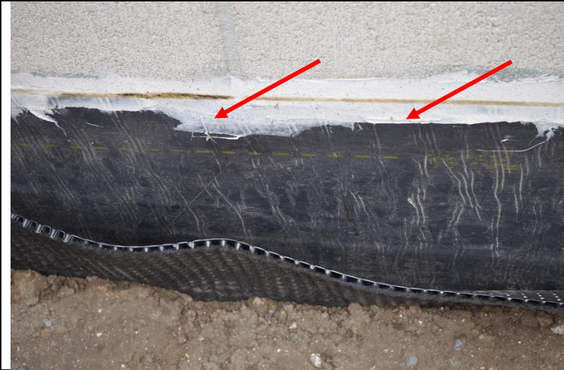
Photo 17: A self-adhered below-grade waterproofing membrane was installed low on the wall. Photo provided by LA BoE, DPW, Architectural Division.
