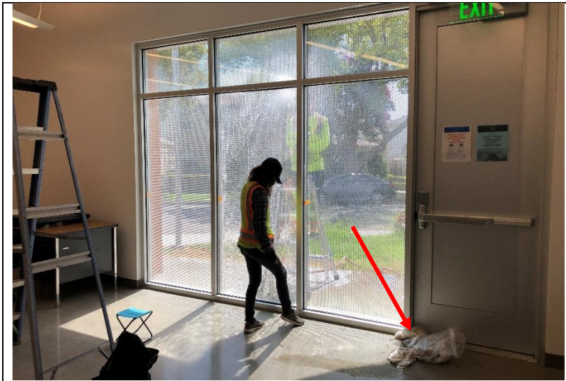
Photo 50: Towels were used to clean up water that entered under the door during diagnostic testing.
