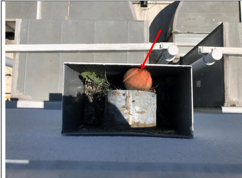
Photo 64: A ball stuck in a scupper drain.
