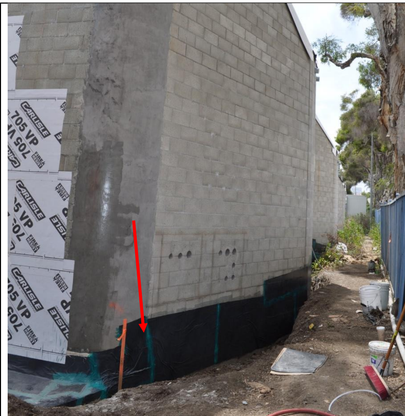
Photo 14: An overview of the east side of the building (during construction). Photo provided by LA BoE, DPW, Architectural Division.
