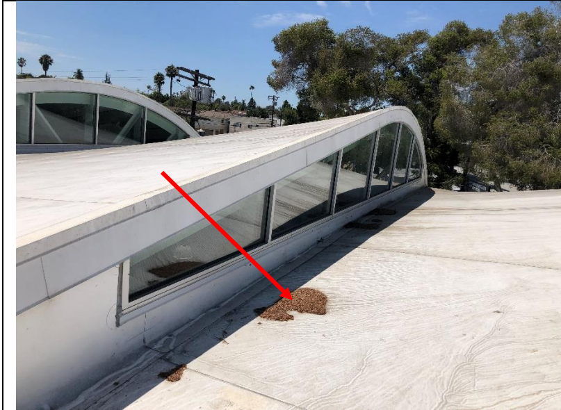
Photo 59: Overview of the ribbon windows on the vaulted roof. Some debris was observed on the roof surface.
