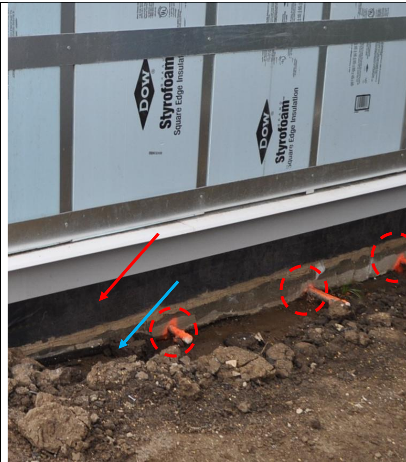
Photo 16: In some locations, the below-grade waterproofing membrane (red arrow) does not appear to be lapped into the methane barrier (blue arrow). Installed in this manner, the vertical edge of the slab is unprotected. Penetrations in this location had not been flashed into the waterproofing system at the time of the photo and (unless corrected) would not be watertight (red circles). Photo provided by LA BoE, DPW, Architectural Division.
