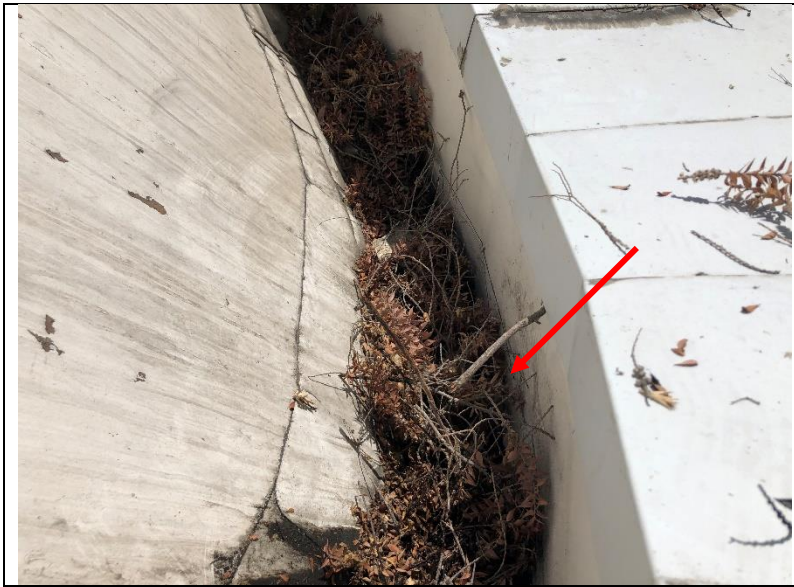
Photo 97: Tree debris built up between the steep slope of the west roof and the low parapet.
