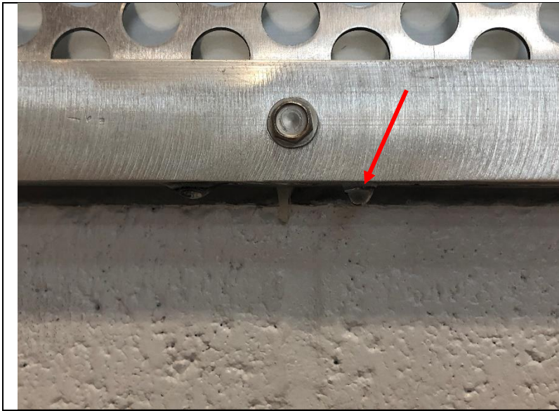
Photo 29: One of the perforated aluminum panel mounting fastener locations leaking during water testing.
