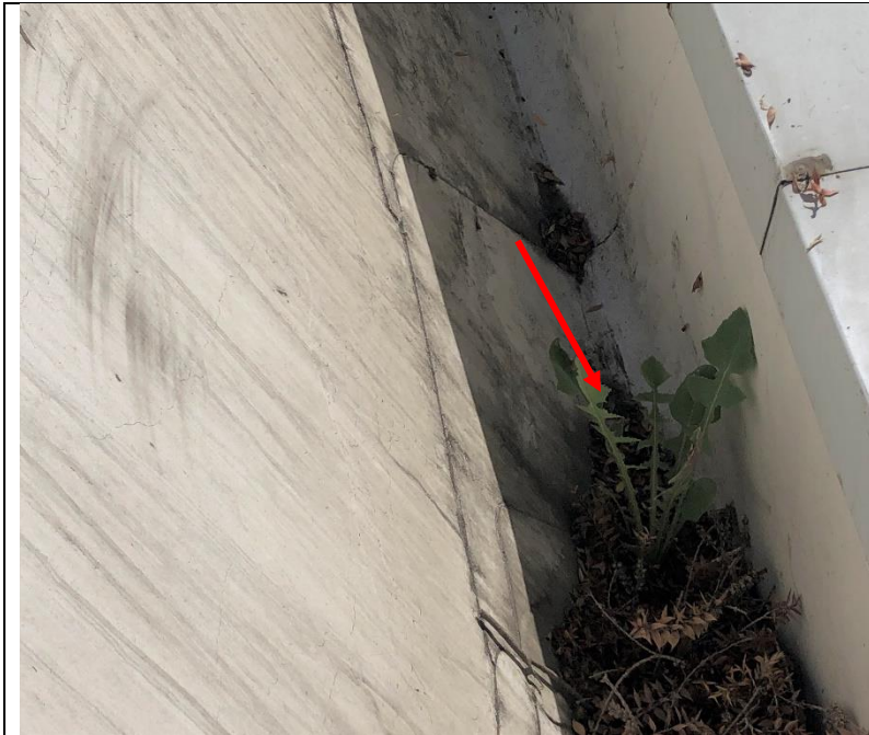
Photo 98: Tree debris built up between the steep slope of the west roof and the low parapet. Plants were observed growing in debris on the roof.
