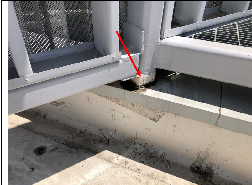
Photo 70: The mechanical curtain supports penetrated the parapet in several locations.
