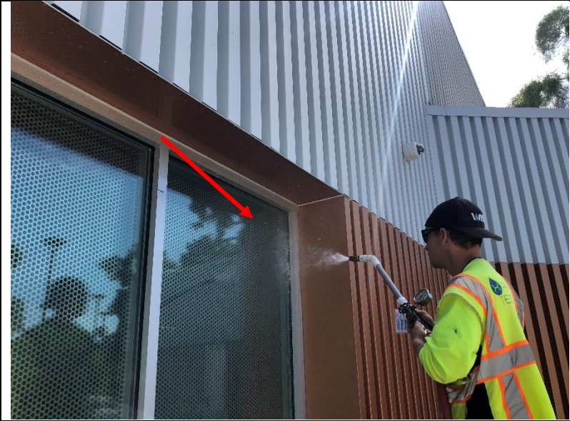
Photo 31: Diagnostic testing at the windows on the south elevation of the indoor basketball court.
