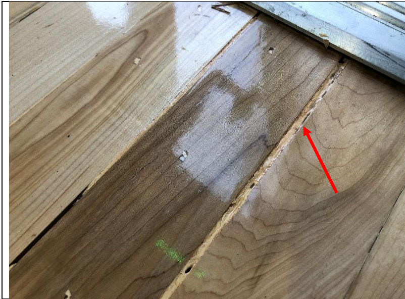
Photo 44: Water damage to the flooring adjacent to the entrance on the south elevation of the indoor basketball court.
