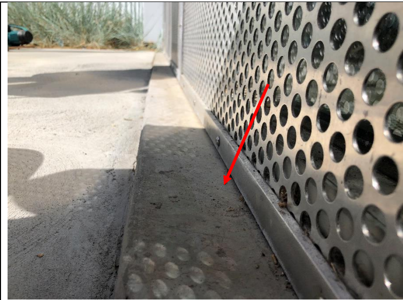
Photo 53: Close view of the storefront at the west entry location, the building slab extends past the bottom of the storefront frame and appears to slope back towards the frame. During water testing water pooled on the slab outside the storefront.
