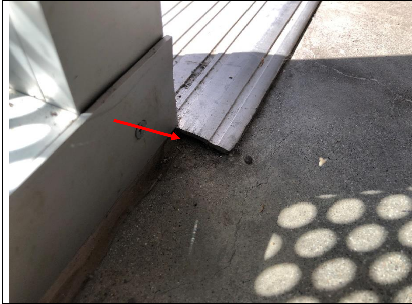
Photo 47: Approved drawings call for a sill pan to be installed under all door thresholds. Sill pans were not observed at any of the door thresholds.
