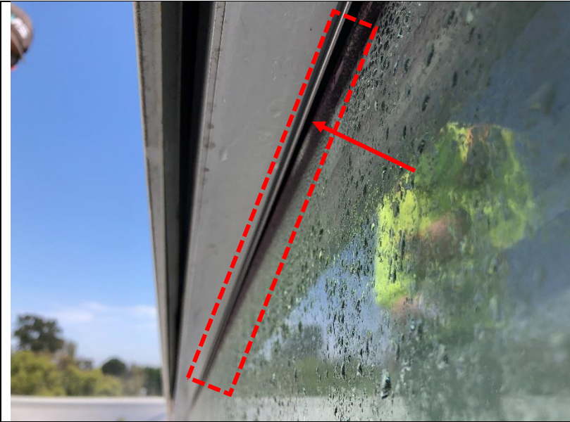
Photo 37: A gasket at the head of one glazing units above the basketball court was missing.
