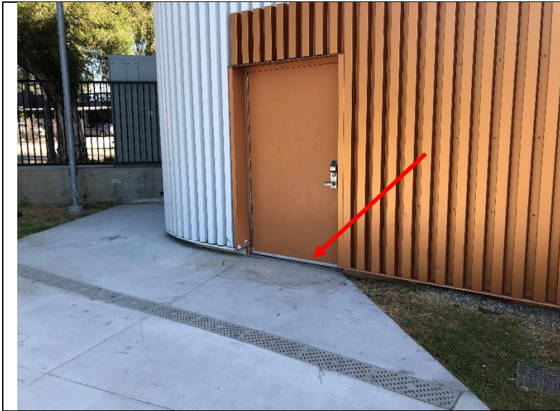
Photo 40: Approved drawings call for a sill pan to be installed under all door thresholds.
