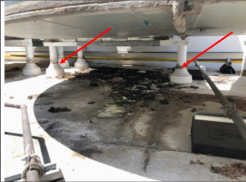
Photo 72: Duct supports also penetrate the roof membrane. Flashings in this view appear to be installed per industry standards.
