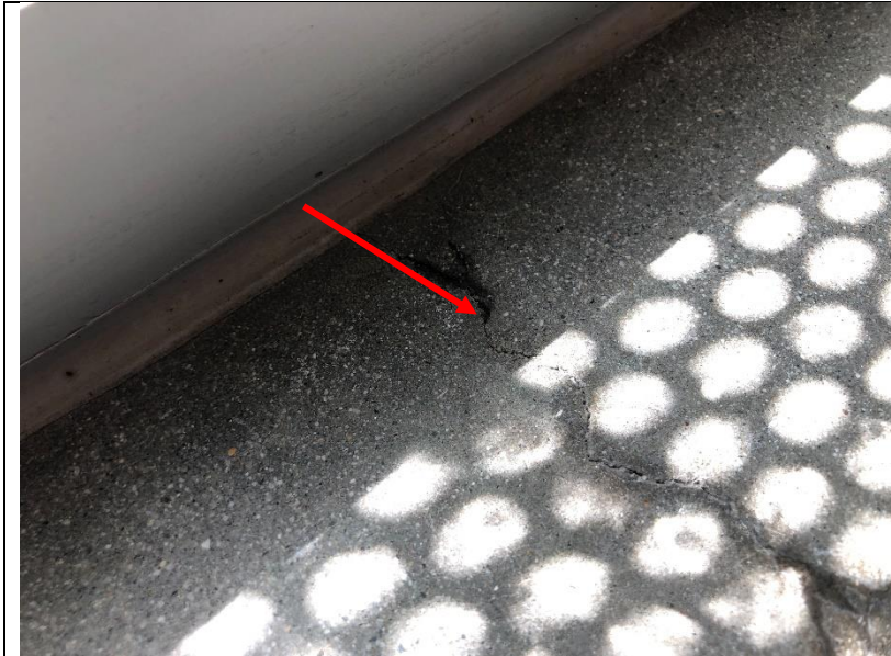
Photo 84: Crack on the interior slab that became wet during testing at the storefront adjacent to the east entry.
