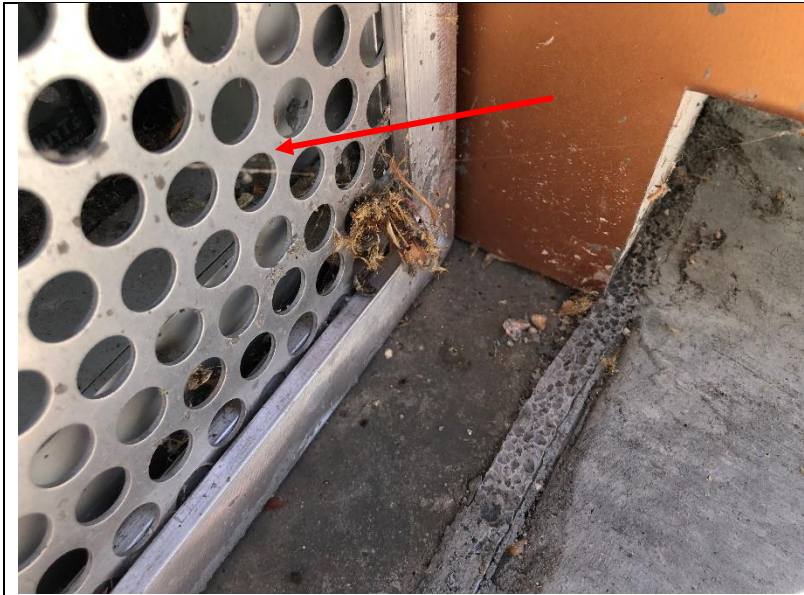
Photo 26: Close-up of a lower corner of a perforated aluminum panel installed at one of the Robertson Recreation Center windows.
