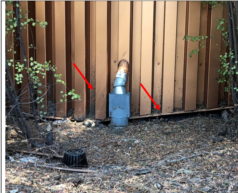
Photo 21: Landscaping debris was visible on the corrugated metal cladding.
