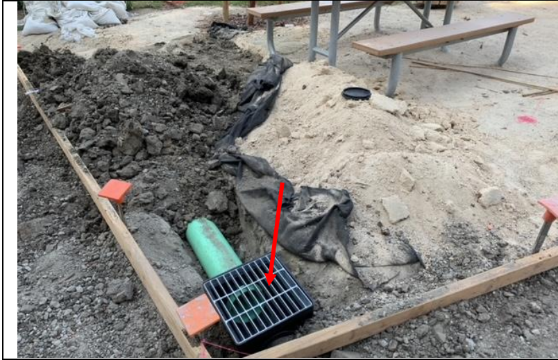
Photo 93: A drain was installed on the south elevation when the sidewalk adjacent to the building was replaced.
