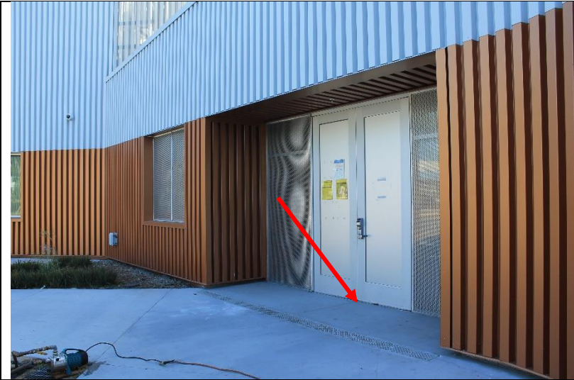
Photo 41: Approved drawings call for a sill pan to be installed under all door thresholds.
