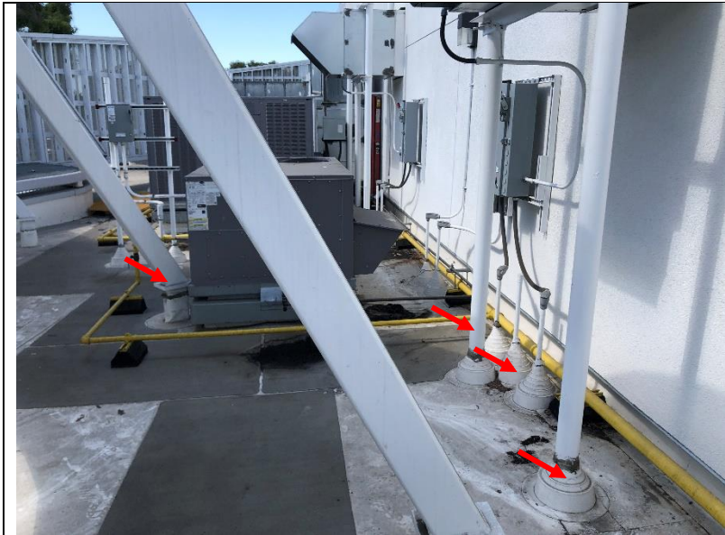
Photo 69: Overview of penetrations on the lower mechanical roof.
