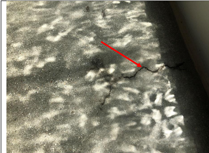
Photo 83: Cracks on the interior slab became wet during testing at the storefront adjacent to the east entry.
