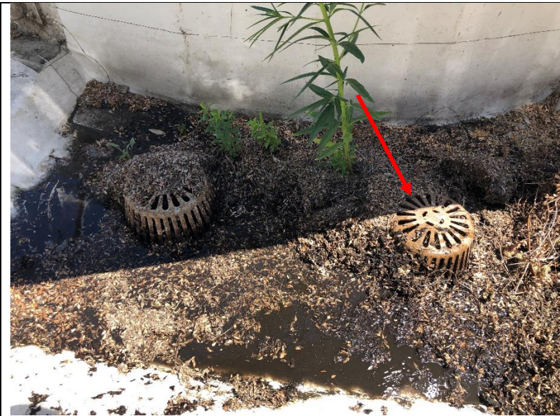
Photo 68: The overflow drain* (red arrow) appears to be lower than the main roof drain.
