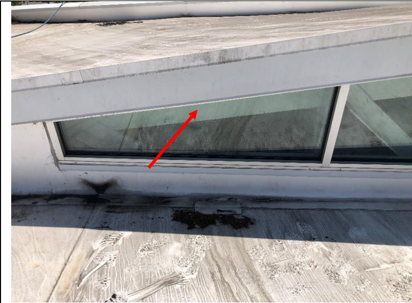
Photo 38: A window with a missing glazing gasket at the head of the window.
