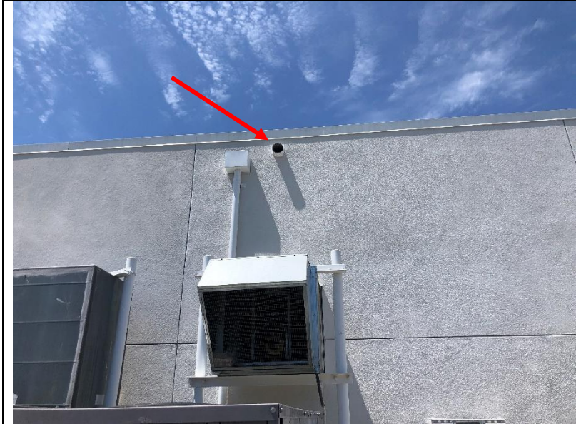
Photo 65: An overflow drain is situated over a ventilation duct.
