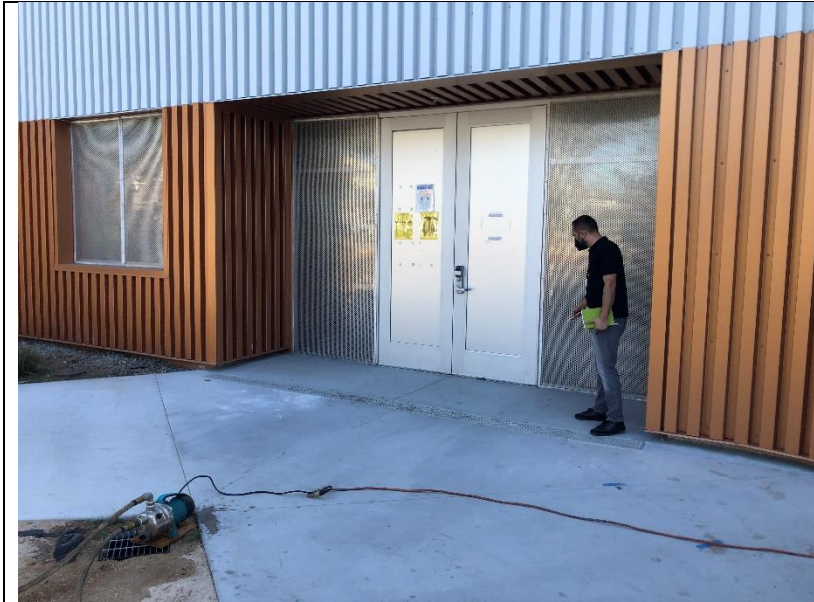
Photo 02: An overview of the corrugated metal panels at the main entrance on the south elevation.
