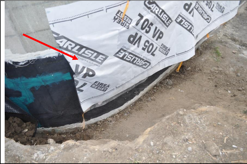
Photo 15: Carlisle 705 VP (an adhered sheet membrane) installed (during construction) on the walls and lapped over the below-grade waterproofing. Photo provided by LA BoE, DPW, Architectural Division.
