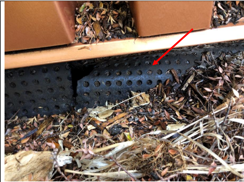
Photo 19: The drain mat was visible below the corrugated metal cladding at some locations. Per the approved drawings, a prefinished 24 gauge galvanized steel flashing with Kynar Coating should have been installed over the drain mat.
