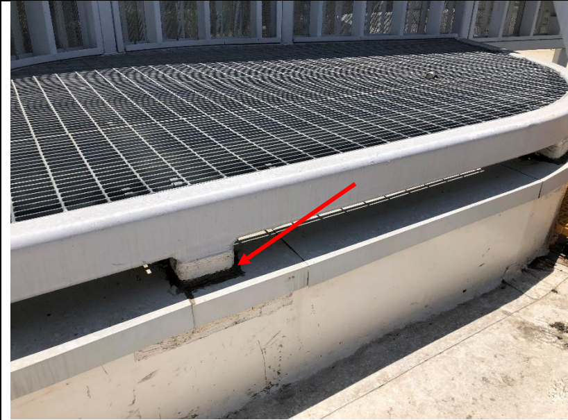
Photo 71: The mechanical curtain supports penetrated the parapet in several locations.
