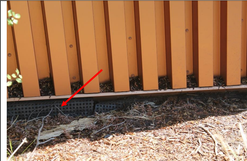
Photo 20: Another location where the drain mat was visible below the corrugated metal cladding. Per the approved drawings, a prefinished 24 gauge galvanized steel flashing with Kynar Coating should have been installed over the drain mat.
