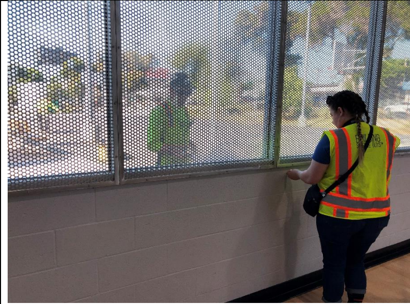
Photo 75: The perforated aluminum panels during diagnostic testing on the south side of the building.
