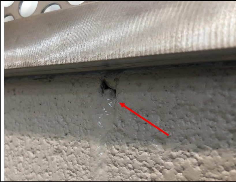
Photo 32: Water seeping from the grout line in a CMU wall below the window sill.
