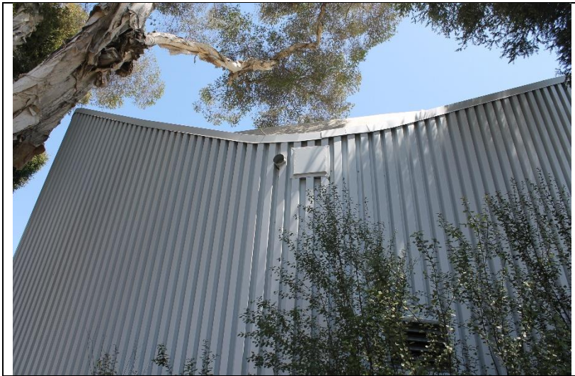
Photo 12: Overview of the corrugated metal cladding system on the west side of the building.
