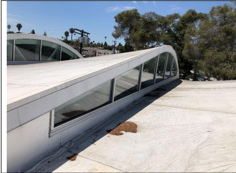
Photo 03: An overview of the upper vaulted roof over the indoor basketball court.
