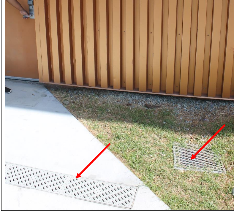
Photo 09: Additional trench drains and area drains had been added in front of and in landscaping adjacent to entrances.
