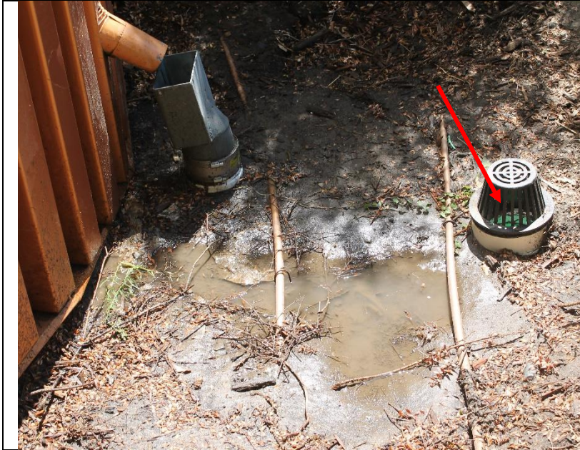
Photo 79: The ground was saturated after diagnostic testing but was not flooded. The surface drain at this location was above grade and not draining the water from the testing.
