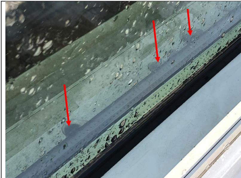
Photo 90: Water was observed at the interior sill of the ribbon windows.
