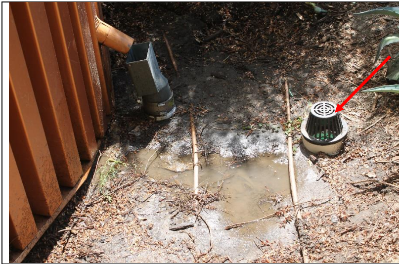
Photo 22: A surface drain that was installed at the same height as the bottom of the corrugated metal cladding.
