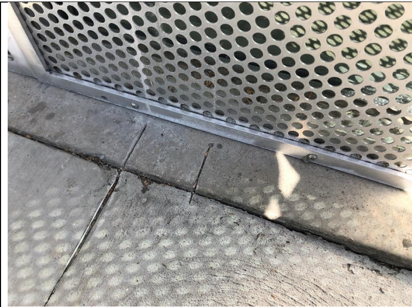
Photo 24: Closer view of the base of some perforated aluminum panels that had been installed at many of the windows.
