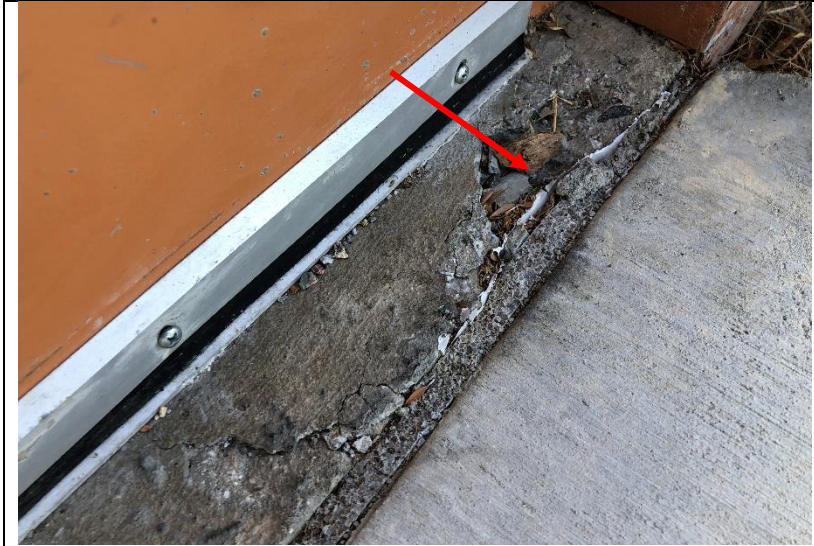
Photo 48: Damage to the concrete surface at a door threshold.
