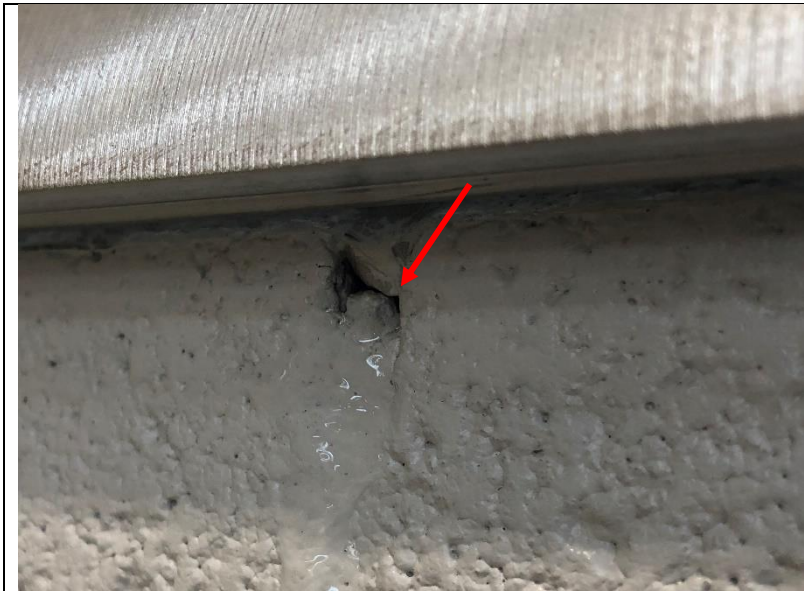
Photo 77: A leak at a grout joint in the CMU wall below the perforated aluminum panels during diagnostic testing on the south side of the building.
