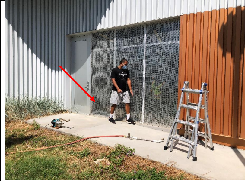
Photo 51: At the storefront and east entry location, the building slab extends past the bottom of the storefront frame to the exterior and appears to slope back towards the frame. During water testing water pooled on the slab outside against the sill of the storefront.
