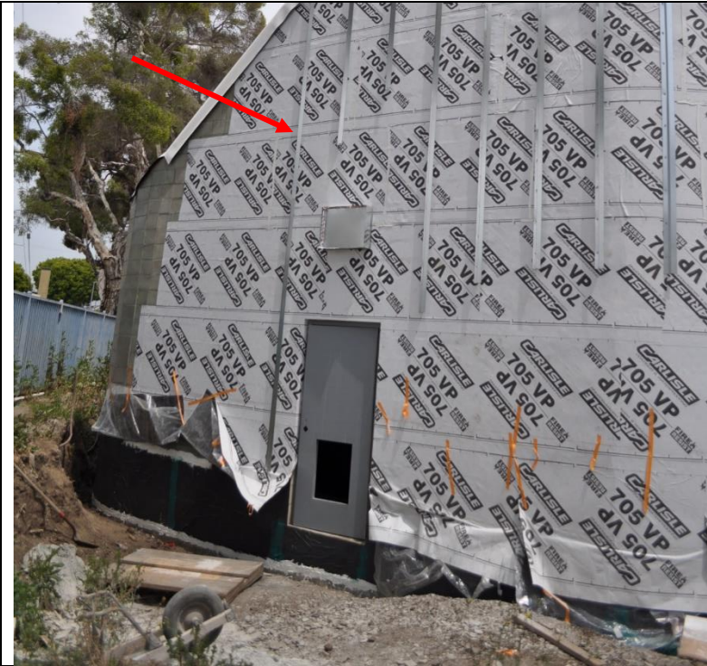
Photo 13: An overview of the west side of the south elevation (during construction) prior to the installation of the corrugated metal cladding system. Photo provided by LA BoE, DPW, Architectural Division.
