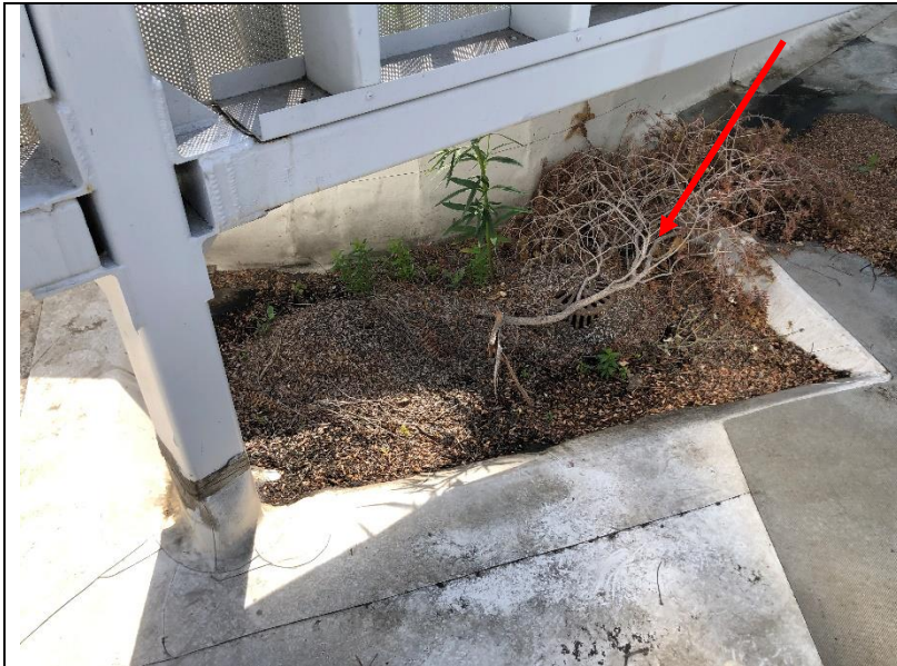
Photo 66: Tree debris filling a lower roof drain recess.
