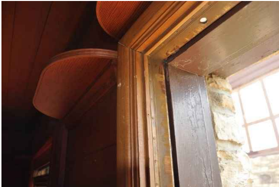
Figure 121: Door trim requires touch-ups.
