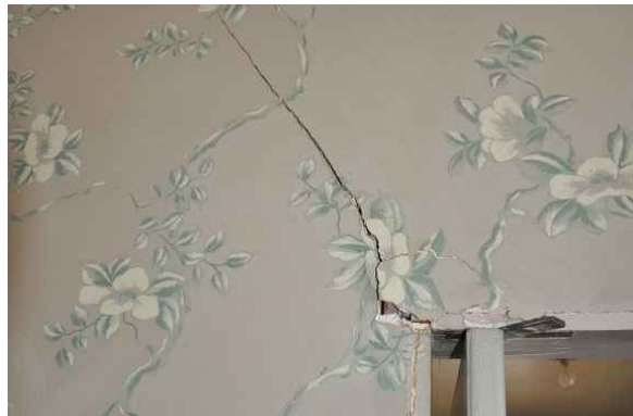
Figure 93: Detail of plaster crack at the west door.
