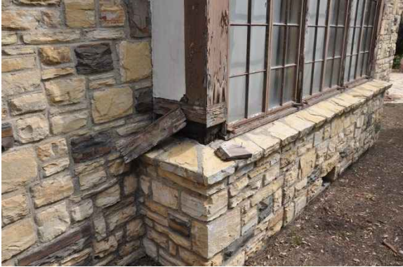
Figure 6: Portions of this wood window surround have detached from the building.
