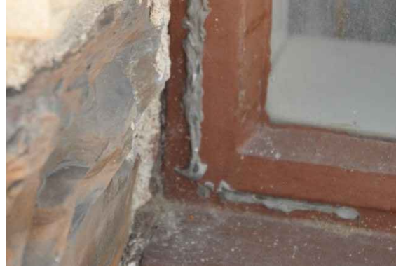
Figure 22: Some sashes have been caulked shut from the exterior and are no longer operable.
