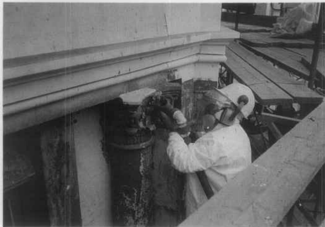
Figure 11. New methods are being developed or adapted to safely remove lead-based paint from various substrates. On this cast iron building undergoing rehabilitation for apartment units, multiple layers of lead-based paint were removed with pneumatic needle guns with vacuum attachments. Paint chips and waste containing lead-based paint were placed in 55 gallon drums for transport to a special waste site, and the workers were fully protected. The cleaned metal was primed and repainted. Photo: Building Conservation Associates, Inc.
