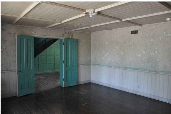
Figure 90: View looking east. Water damage is present at the east wall, floor and ceiling due to plumbing leak.
