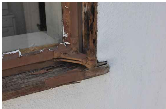
Figure 24: Glazing compound is typically cracked and wood sills require repair (see exterior wood section).
