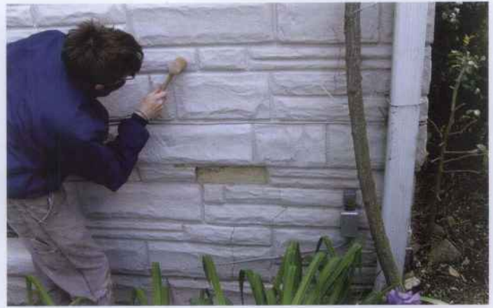
Figure 6. Stucco applied to an exterior wall or foundation was intended to function as a watertight surface. Unless maintained, rainwater will penetrate open joints and cracks that may occur over time. A spalled section of stucco indicates some damage has occurred and a wooden mallet is being used to tap the surface to determine whether the immediate stucco has lost adhesion. Photo: Bryan Blundell.
