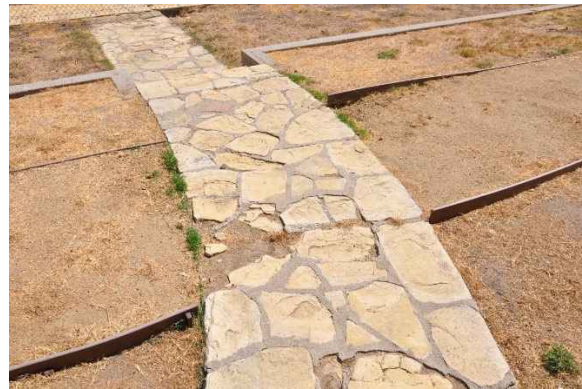
Figure 65: The flagstone paths throughout the yard zone require repair.
