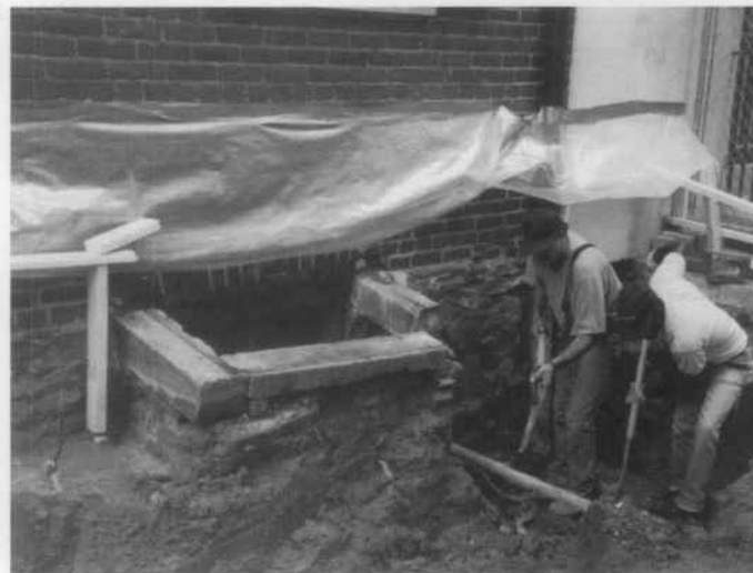
Fig. 5. Excavating this foundation revealed that the downspout pipe had corroded at the “u-trap” and was leaking moisture into the soil. Openings around the horizontal water supply line and cracks in the wall allowed moisture to penetrate the basement in multiple locations. Photo: author.
