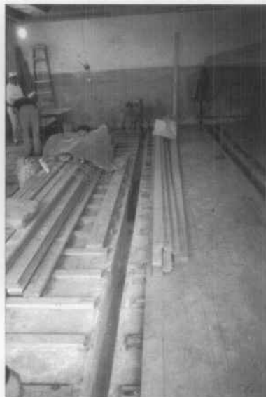
D. In a flood plain, rotted joists were replaced with a concrete slab and sleepers designed to drain water. Spaced flooring allowed drainage and room for damp wood to swell without buckling. Harper's Ferry Center, NPS.
