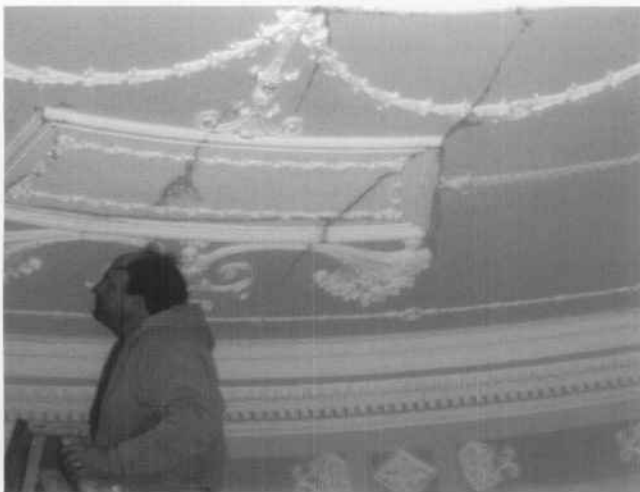
Fig. 6. Uninsulated plumbing pipes close to the exterior wall froze and cracked, wetting this ornamental plaster ceiling before the water supply line could be shut off. As a result, limited portions of the ceiling needed reattaching. Photo: author.
