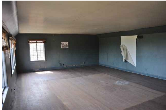
Figure 132: View of the room today from a similar angle looking west. Wallpaper is delaminating significantly.
