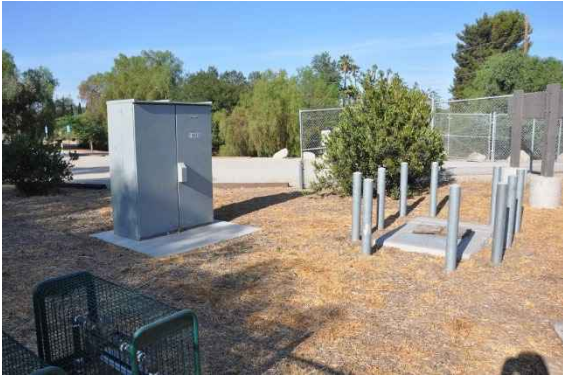
Figure 54: View of the updated transformer and switchgear along Devonshire.
