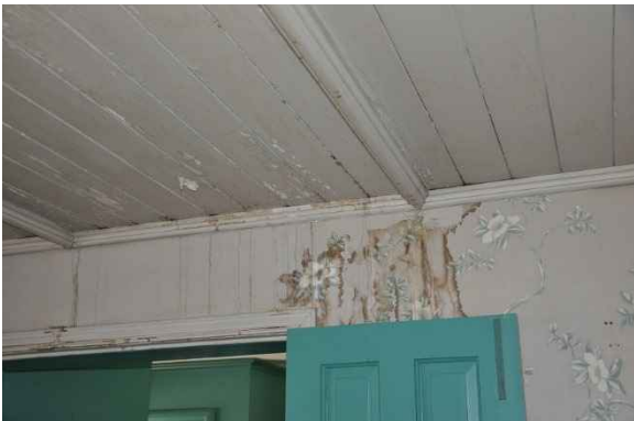
Figure 92: Detail of water damage at the east door.
