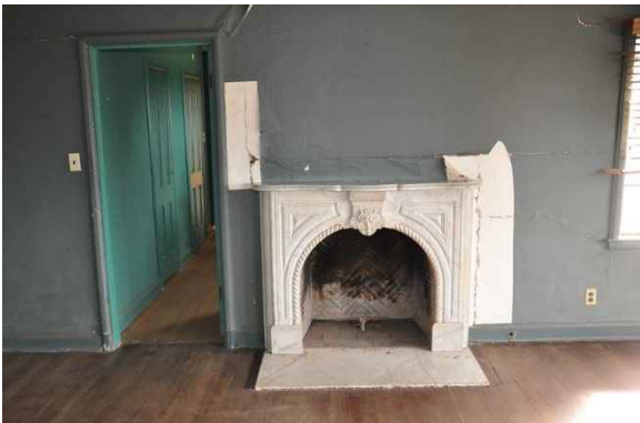
Figure 135: Original marble fireplace surround and adjacent cracked plaster wall with delaminating wallpaper.
