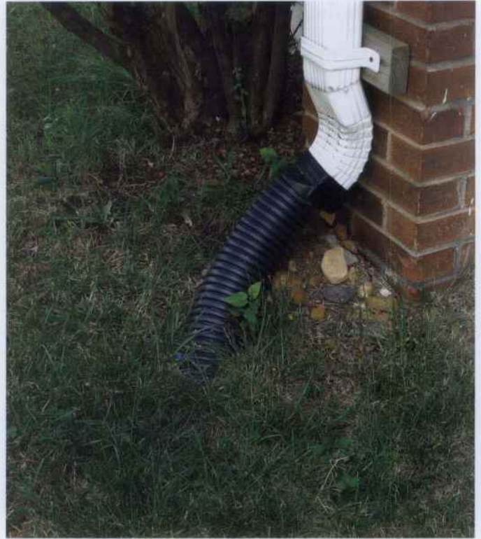
Figure 17. Extending downspouts at their base is one of the basic steps to reduce dampness in basements, crawl spaces and around foundations. Extensions should be buried, if possible, for aesthetics, ease of lawn care, and to avoid creating a tripping hazard. Photo: NPS files.
