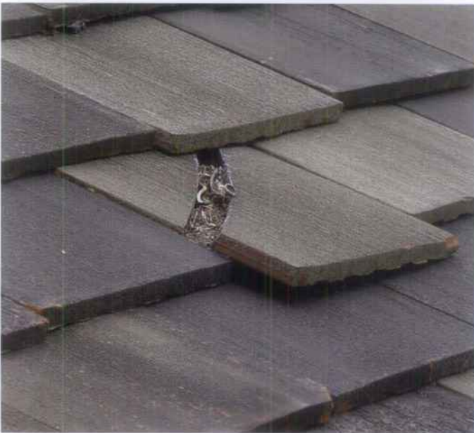
Figure 4. Damage to roofs often requires immediate attention. As a temporary measure, this damaged roof tile could be replaced with a brown aluminum sheet wedged between the existing tiles. Photo: Chad Randl.
