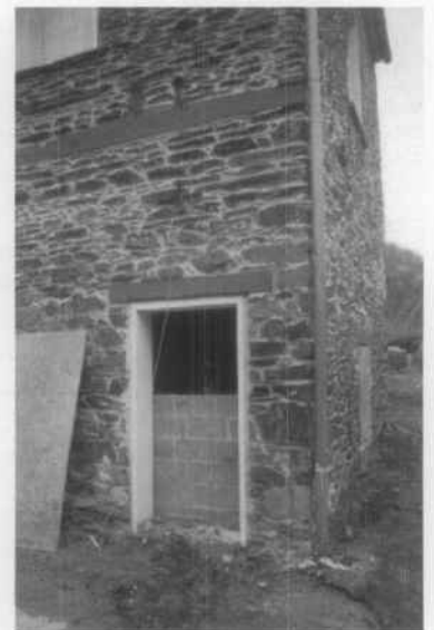
E. Mechanical systems on the lower level were placed on platforms above the flood line. Harper's Ferry Center, NPS.
