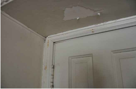
Figure 42: Thick layers of flaking paint have chipped and fallen away from plaster in some areas.
