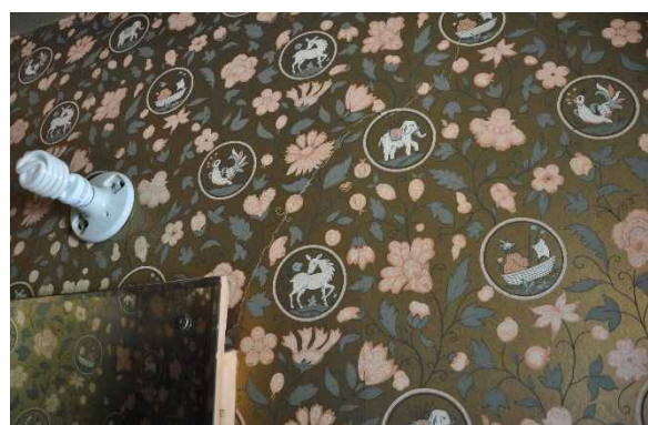
Figure 47: Ornate wallpaper remains in the Powder Room.
