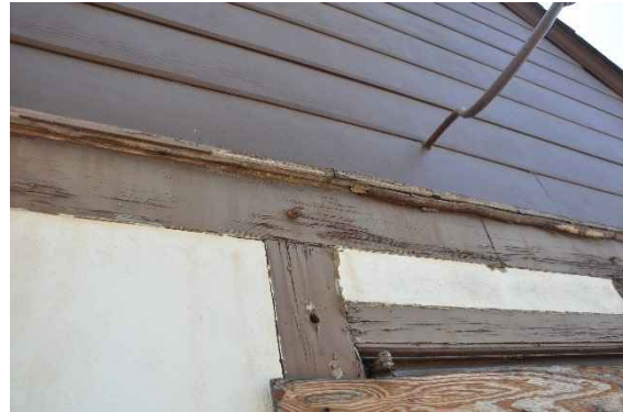
Figure 9: Flaking paint, wood deterioration and missing pegs at west garage facade.
