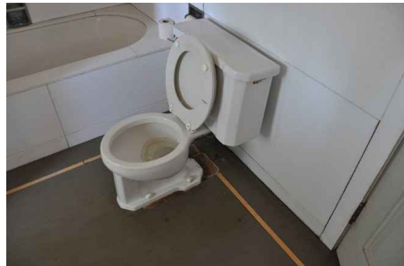
Figure 114: Original linoleum floors remain, and some repair is required.
