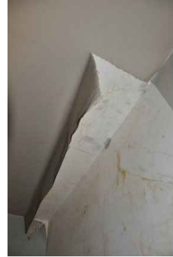
Figure 112: Peeling wallpaper at the vestibule.
