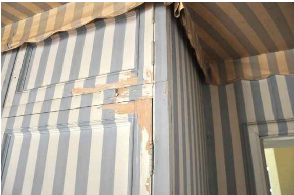
Figure 140: Detail of striped wall paint requiring touch-ups.
