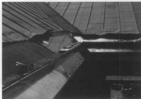
B. Repair roofs and add ice and water shields at eaves and under valleys in cold climates. Photo: Larry D. Dermody.
