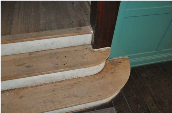
Figure 36: The first two stair treads at the entry hallway have exposed plywood subfloor with carpet tack holes and some discoloration.
