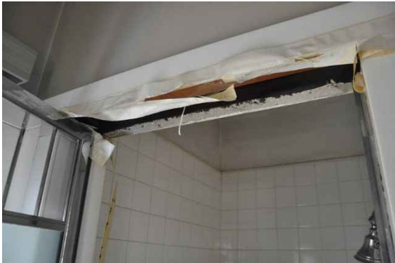
Figure 115: The shower door header requires repair.
