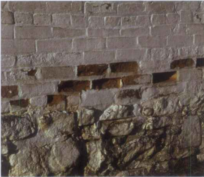
Figure 10. Repointing of masonry should usually be approached as repair rather than maintenance work in part because of the need for a skilled mason familiar with historic mortar. In this case, a moisture condition was not corrected and the use of a waterproof coating and off-the-shelf Portland cement mortar trapped water and resulted in further damage to these 19th century bricks. Photo: NPS files.
