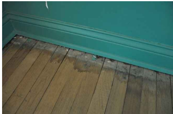
Figure 37: Water damage is present at floor boards in the second-floor corridor.
