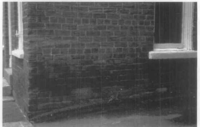
Fig. 11. Capillary rise of moisture in masonry is often accompanied with a horizontal tide-mark line several feet above the grade, as seen here. Removing or redirecting as much ground moisture as possible usually helps reduce moisture within a wall. Photo: NPS Files.
