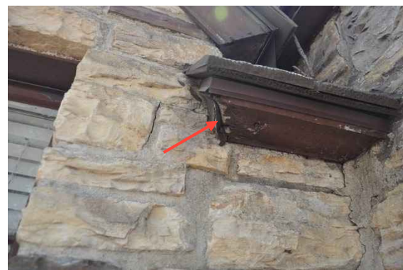
Figure 5: Eave trim is separating at corner joints in some areas.
