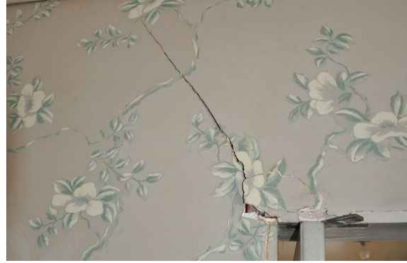
Figure 43: Wallpaper has ripped over cracking at plaster, often at corner joints.
