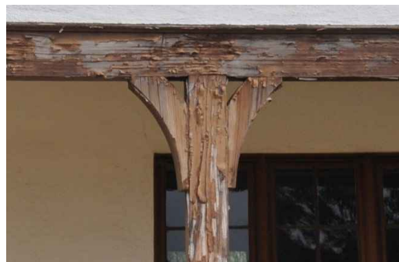
Figure 14: Detail of knee brace with extensive flaking paint.
