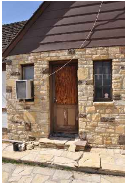
Figure 28: The door leading into one pool restroom is boarded where a large portion of panel was removed.
