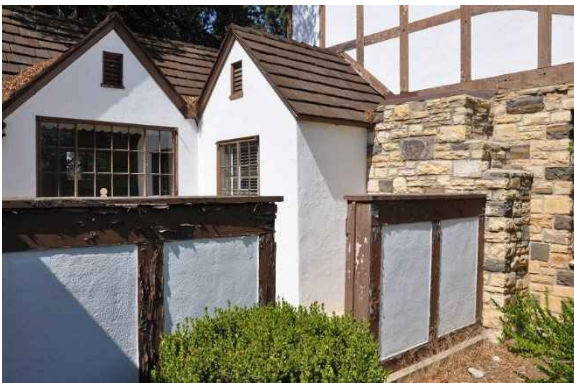
Figure 12: Wall at drying yard is not structurally sound and requires repairs using in-kind materials to match the existing wall.
