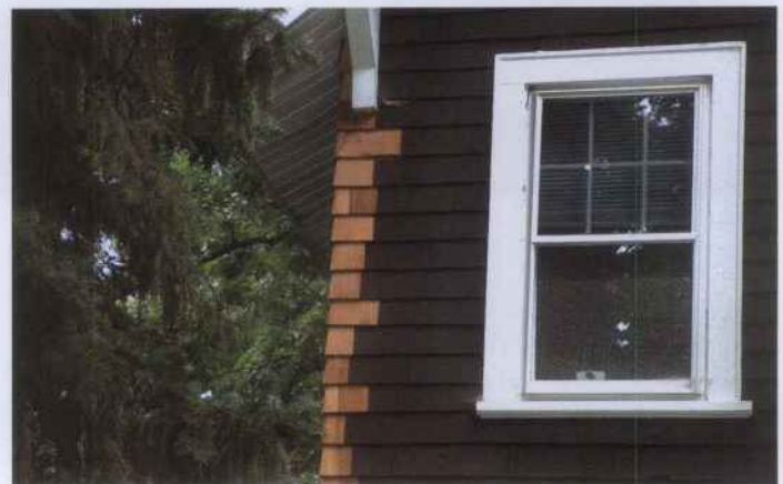
Figure 7. One of the advantages of wood shingles as a wall covering is that individual shingles that are damaged can easily be replaced. On this highly exposed corner, worn shingles have been selectively replaced to help safeguard against water damage. The new shingles will be stained to match the existing shingles.
