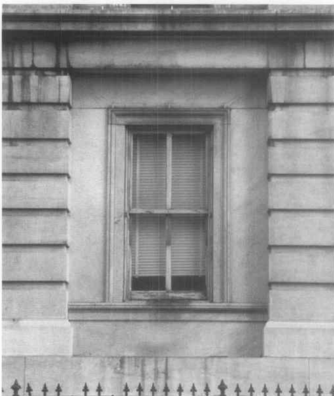
Fig. 10. Infiltration of damp air can occur around loose-fitting or deteriorated window sash and through cracks or open joints in building exteriors. Photo: Ann Brooks Prucher.
