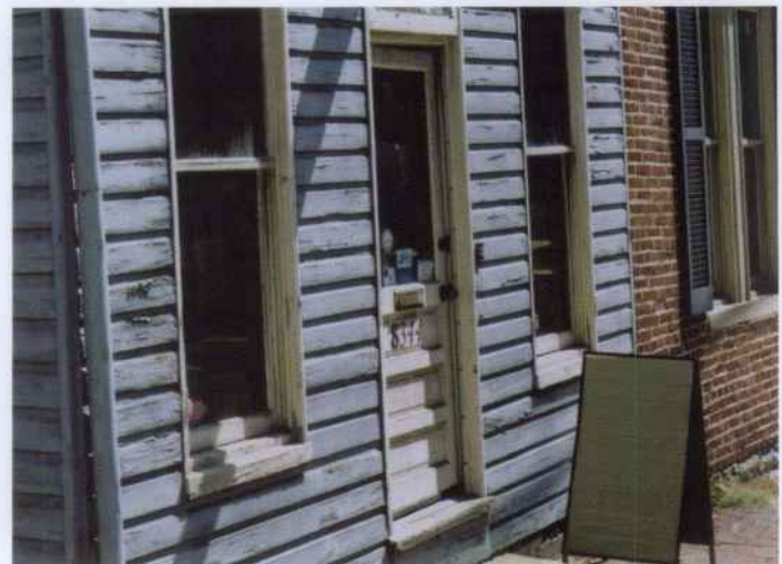
Figure 8. The paint on the siding of this south-facing wall needs to be scraped, sanded, primed and repainted. Postponing such work will lead to further paint failure, require greater preparatory costs, and could even result in the need to replace some siding. Photo: Charles Fisher.
