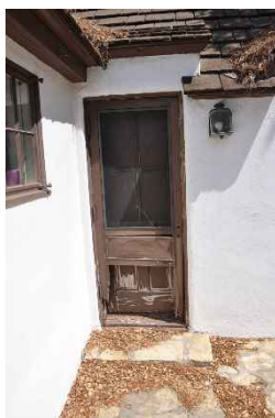
Figure 26: The screen door leading into the drying yard requires reconstruction.
