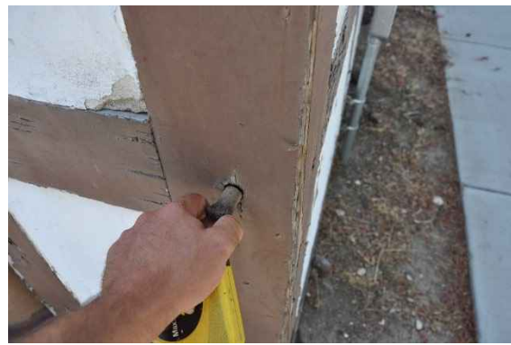
Figure 11: Loose peg at northwest corner of garage.
