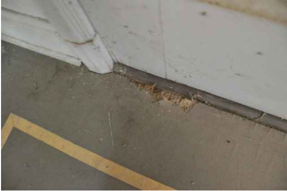
Figure 111: Linoleum with frayed fibers at the vestibule threshold.
