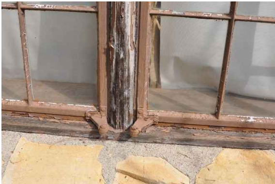
Figure 23: Window paint at exterior is generally deteriorated.
