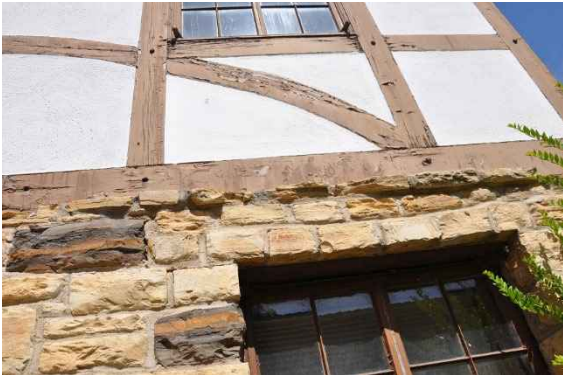
Figure 8: Flaking paint, wood deterioration and missing pegs at south second floor façade.
