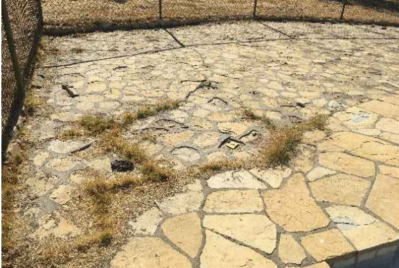
Figure 68: View of the flagstone pool surround showing deterioration and unwanted plant growth.
