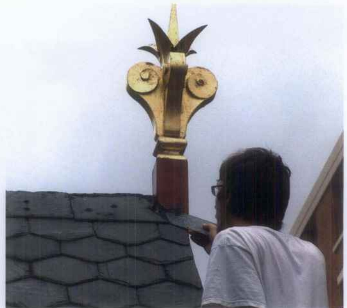
Figure 5. The use of a sealant to close an exposed joint is not always an effective long-term solution. Where this decorative wood element connects to the slate roof, the sealant has failed within a short time and a proper metal flashing collar is being fitted instead. Photo: Bryan Blundell.
