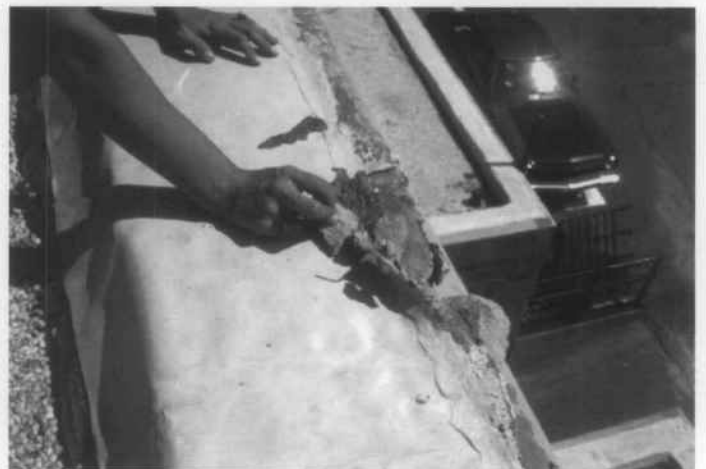
Fig. 1. Moisture problems, if not properly corrected, will increase damage to historic buildings. This waterproof coating trapped moisture from the leaking roof, causing portions of the masonry parapet to fail. Photo: NPS Files.
