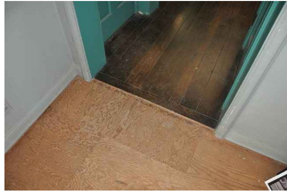
Figure 41: The plywood subfloor is exposed in the living room and guest wing bedroom where finishes have been removed.
