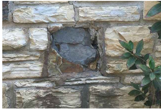
Figure 20: Dark sandstone has spalled and is missing pieces.
