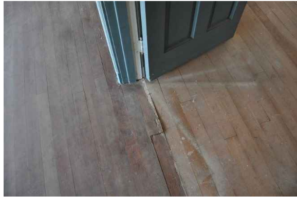
Figure 35: Loose boards at this room threshold should be reattached.
