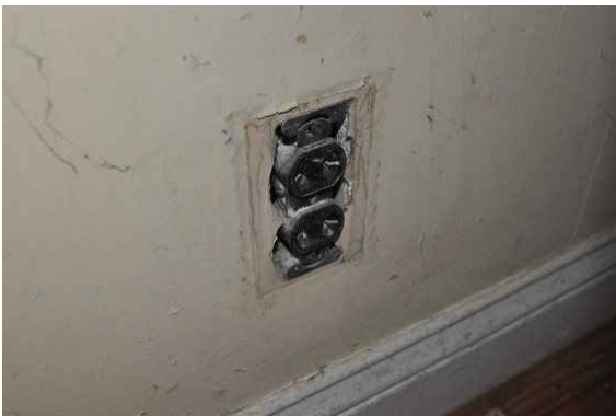
Figure 56: Many electrical outlets require repair.
