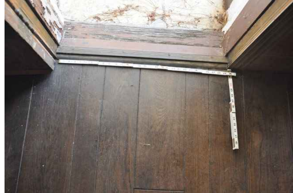
Figure 60: Door threshold leading from the south porch into the Great Room, which may require only minor modification to meet Historic Building Code accessibility standards.
