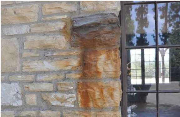
Figure 17: Dark sandstone is leaching iron onto surrounding limestone at north façade, creating dark orange streaks.
