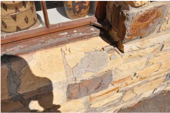
Figure 19: Limestone is flaking at horizontal surfaces.
