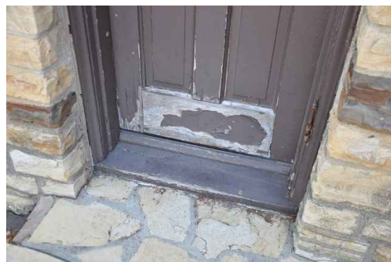
Figure 27: Lower portions of doors typically show more advanced deterioration.
