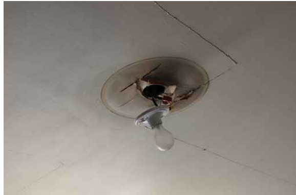
Figure 57: Light fixtures throughout the house have been damaged and likely require rewiring in order to restore operability.
