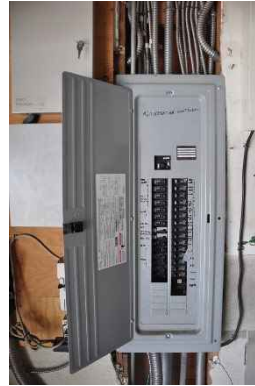
Figure 55: A new electrical subpanel was installed in the garage but the connection to new service was not completed.
