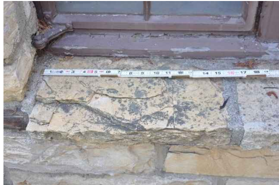
Figure 18: Limestone has discolored patches from environmental accumulation at horizontal surfaces such as window sills.
