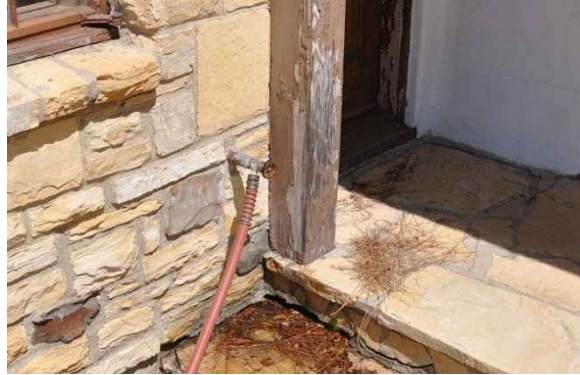
Figure 16: Pier base requiring paint repair.
