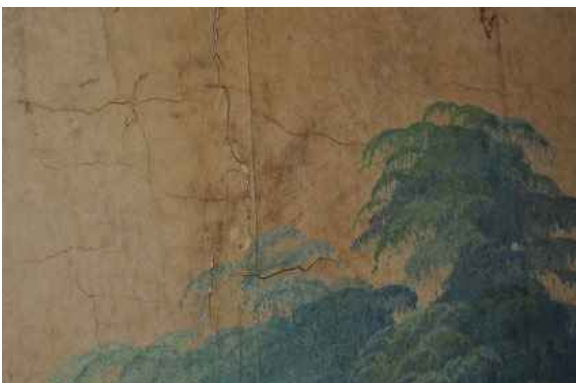
Figure 46: The Great Room wallpaper murals have cracked and discolored over time, likely due to heat and sun exposure.
