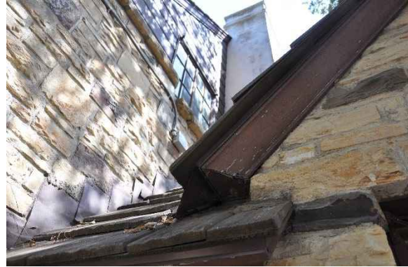
Figure 7: Rake boards typically require a new coat of paint.
