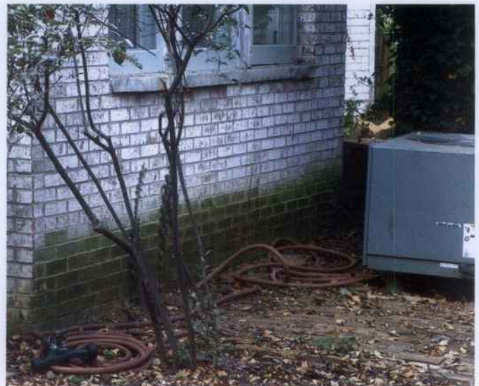
Figure 16. This chronically wet area has a mildew bloom brought on by heat generated from the air-conditioning condenser unit. The dampness could be caused by a clogged roof gutter, improper grading, or a leaking hose bibb.
