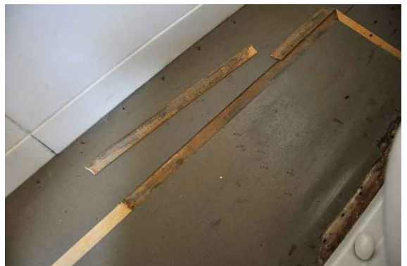
Figure 39: Detail of linoleum accent strips which have delaminated from the subfloor.
