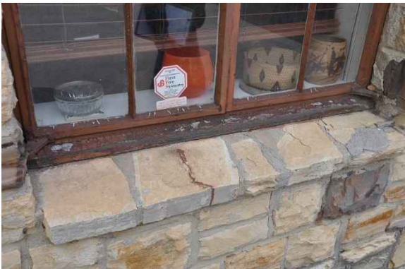
Figure 4: Wood sills typically require patching and paint.
