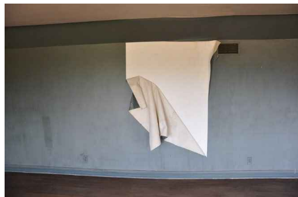
Figure 45: Large swaths of wallpaper have delaminated in some areas.
