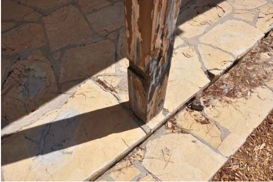
Figure 15: Damaged pier base with missing material.
