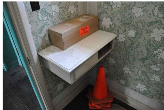
Figure 87: Phone room millwork requires repair.
