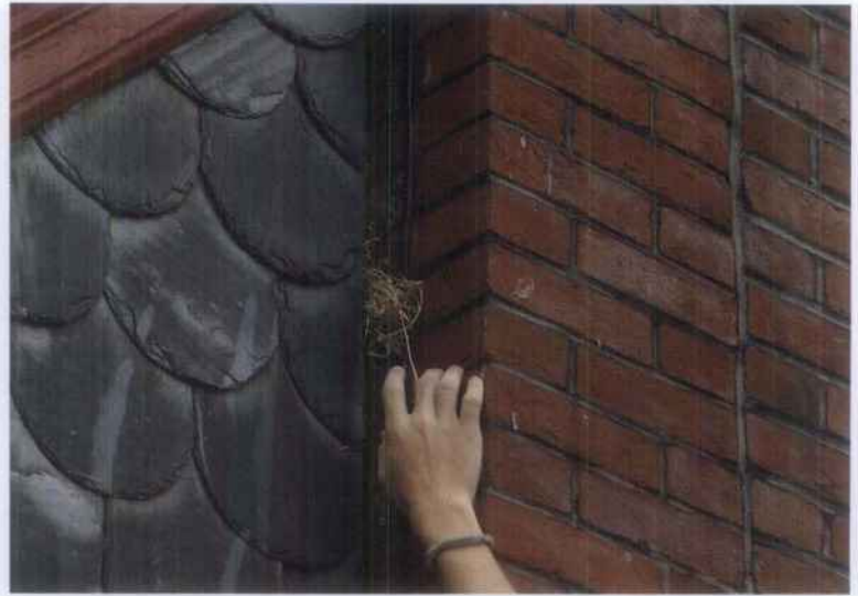
Figure 14. When inspecting connections between projections and the main building, look for areas where birds, bees and pests may enter or nest. Birds have been nesting in this porch roof and the area is being cleaned of their debris. Where an opening exists, it may be necessary to cover it with a trim piece, screening, or sealant. Photo: Bryan Blundell.
