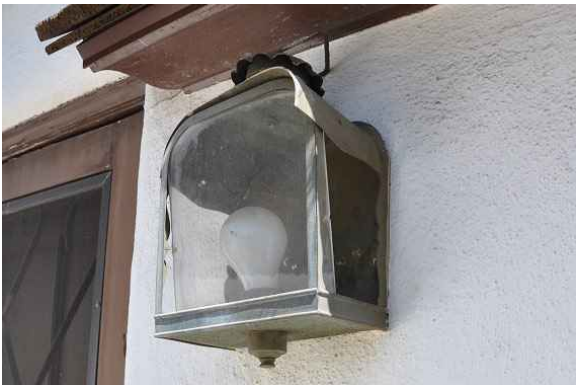
Figure 32: original light fixture at the south kitchen entry to be refurbished.
