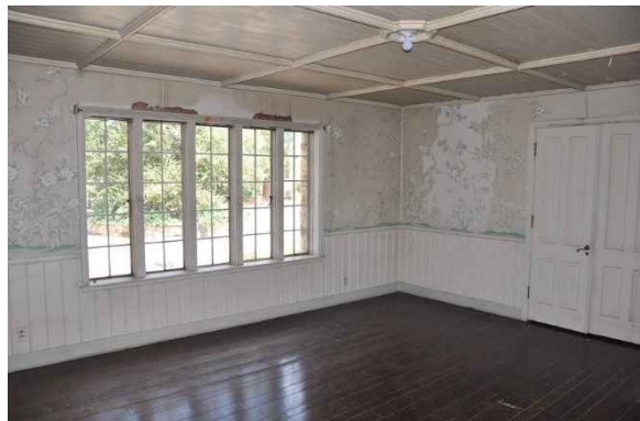
Figure 91: View looking north. Water damage is present above the windows.
