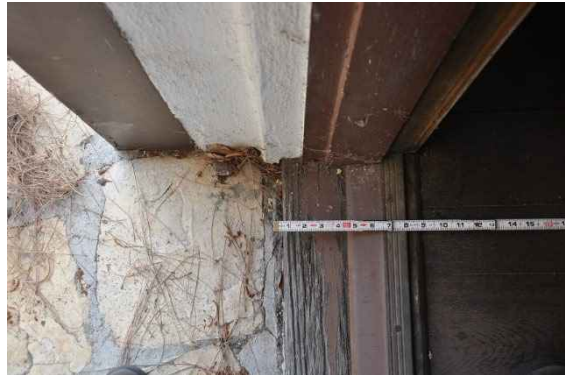
Figure 29: Exterior wood sills are typically deteriorated, and many require replacement.
