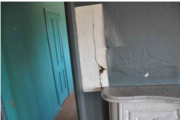
Figure 44: Typical plaster cracking condition.
