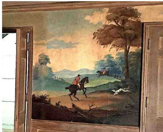
Wall with the most unstable paper adhesion (area of past water leakage?)
