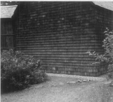
C. The new ground gutter gravel base helps drainage around the concrete foundation (see B above) which is not visible behind the replaced wooden wall shingles. Photo: WPTC, NPS.
