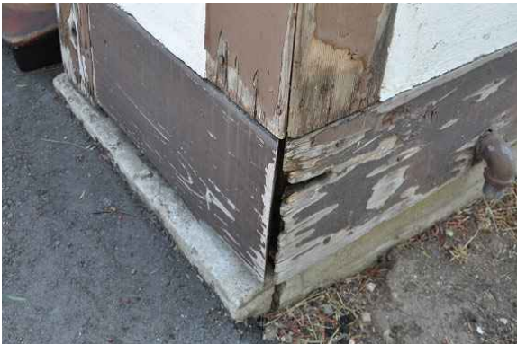
Figure 10: Deteriorated boards separating at northwest corner of garage.
