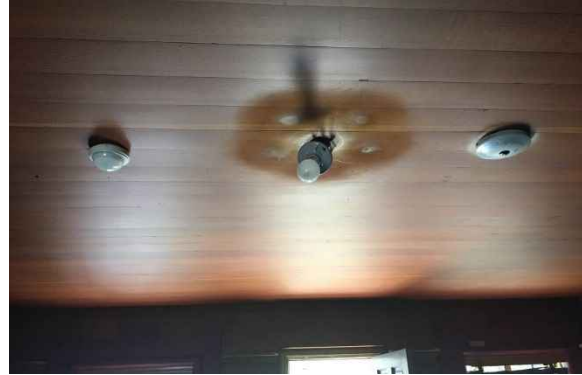
Figure 51: The Trophy Room ceiling bares evidence of a missing light fixture.
