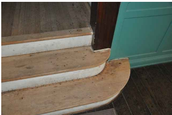
Figure 86: First two stair treads require repair.
