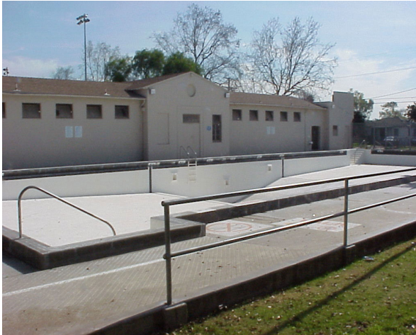
109 th Street is an important resource in the community, but needs to be replaced
