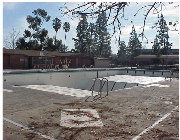
Valley Plaza needs to be replaced.
