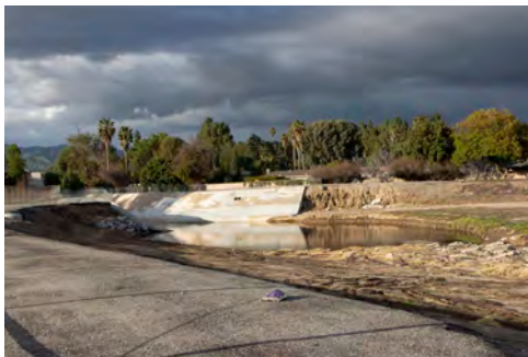
Wilbur Debris Basin
